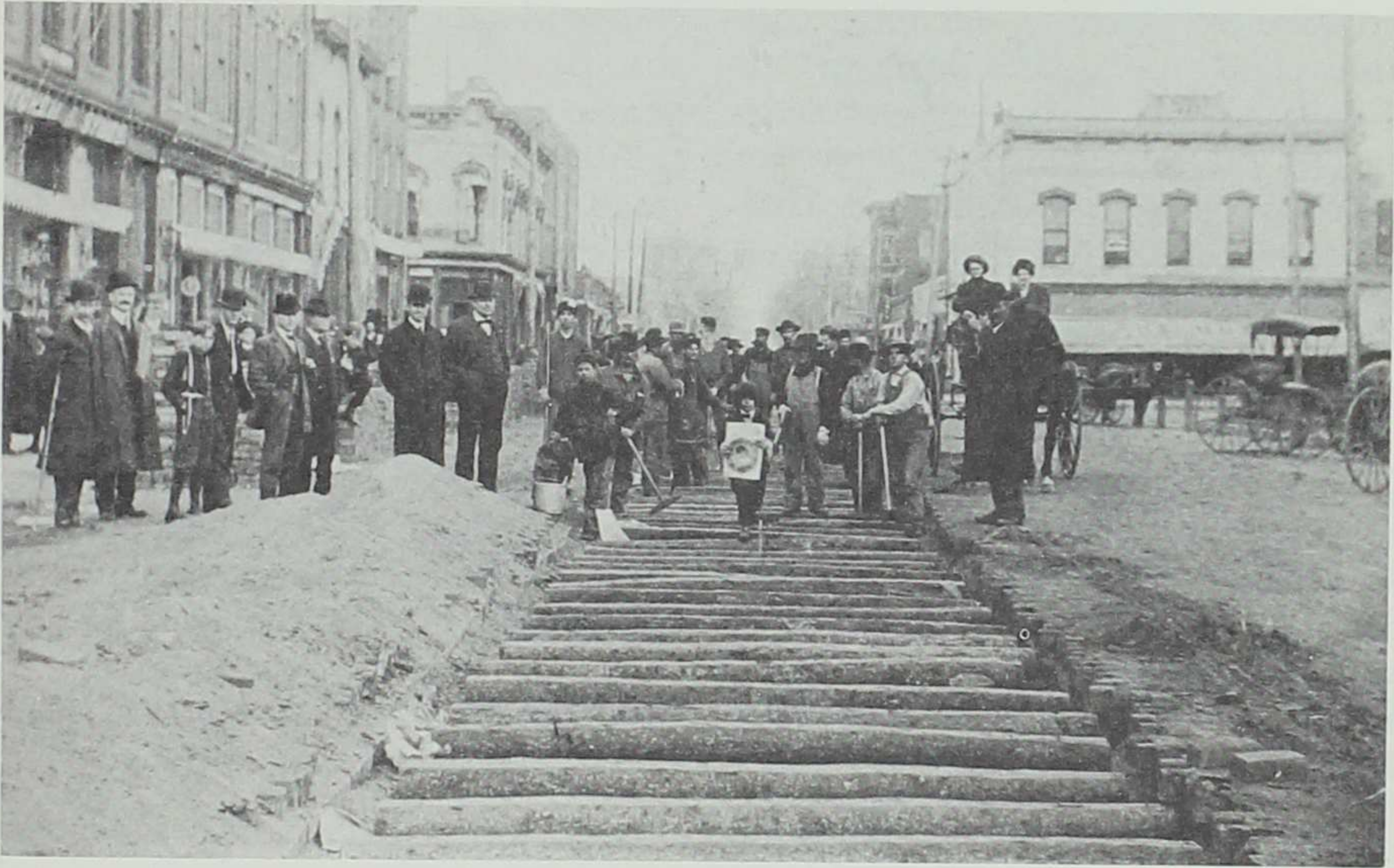
Ceremonies in the Spring of 1907 on the west side of the public square in Albia to mark the construction of the Albia to Hocking line of the Albia Interurban (courtesy of Mrs. W. A. Magie, Albia).
