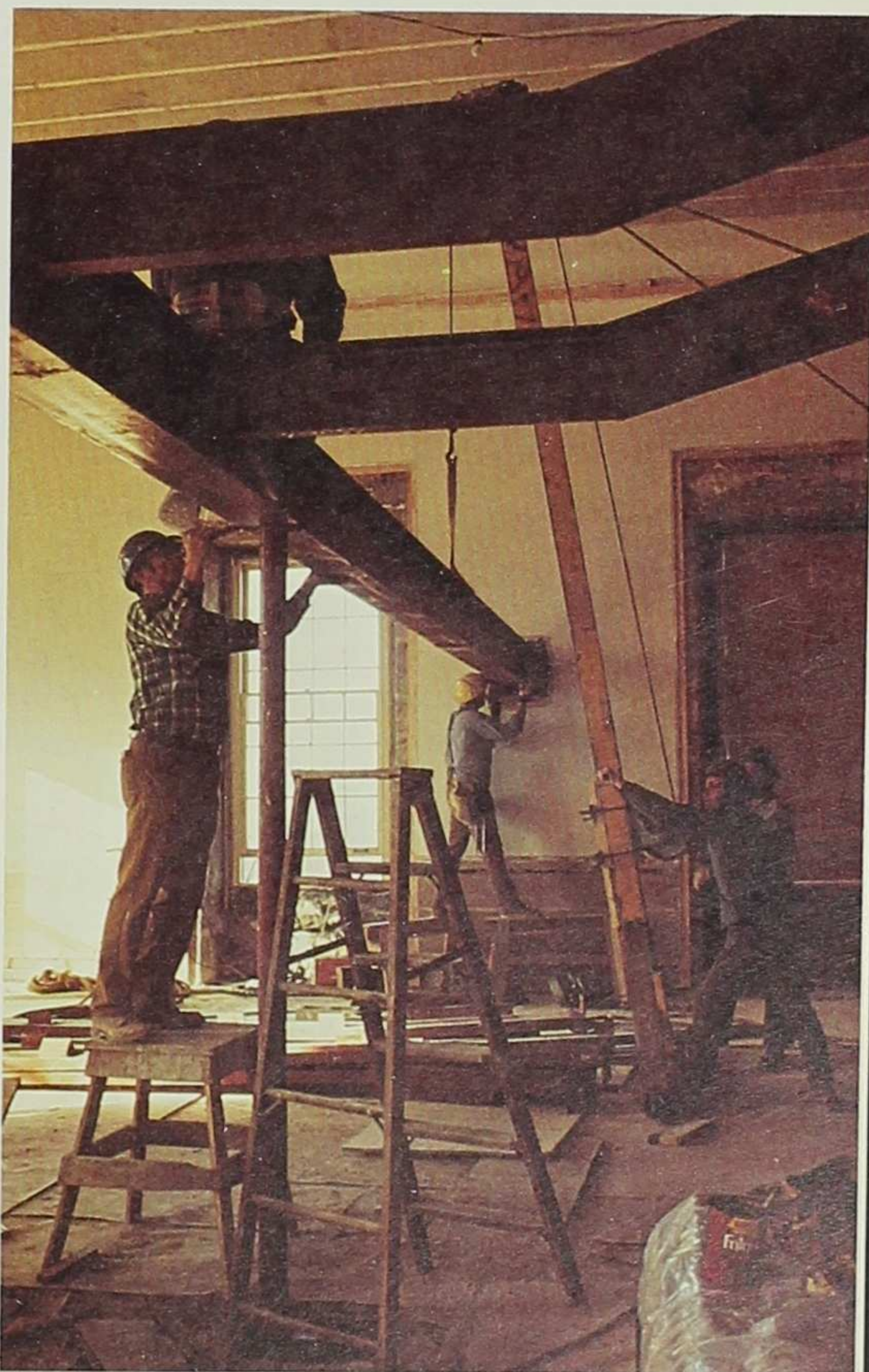
Workmen install steel support beams for the gallery in the House Chamber in November 1974. (courtesy of The University of Iowa, Don Roberts photo)
