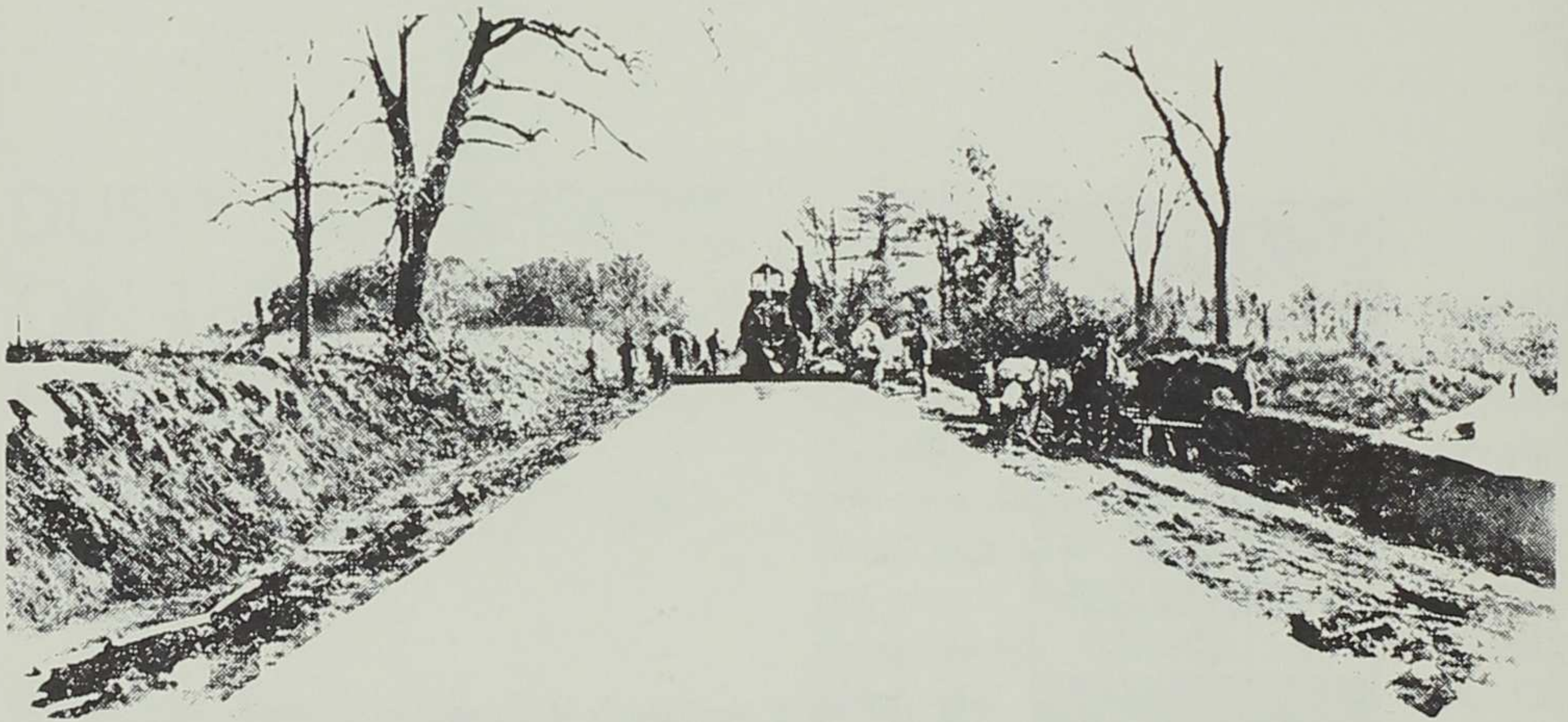
The concrete "Seedling Mile" under construction in Linn County near Cedar Rapids in 1918. The Portland Cement Association provided materials free of charge (Lincoln Highway Association photo).
