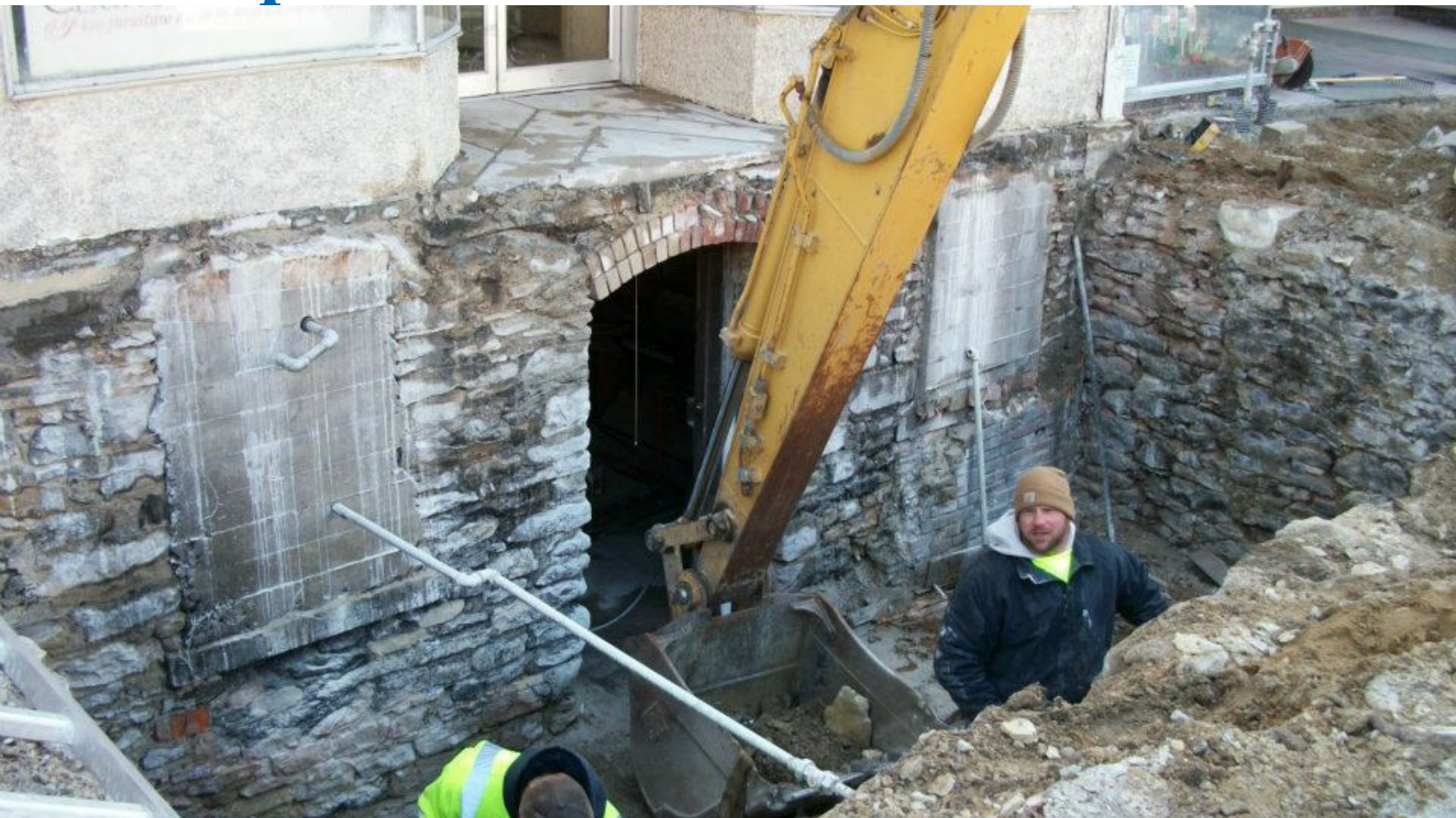
Underground Sidewalk Project, South Side of 1st Street. Article photos courtesy of Leanne Harrison.
