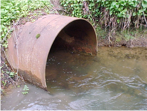
Before – 4 foot CMP
