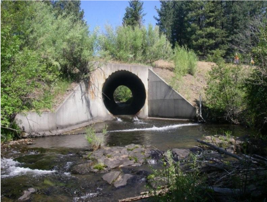
Before – 10.5 foot CMP
