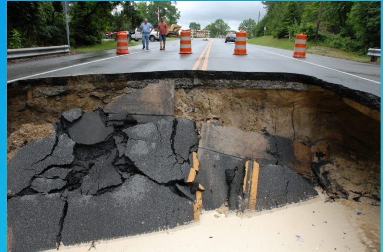
Culvert Collapse - Sussex
