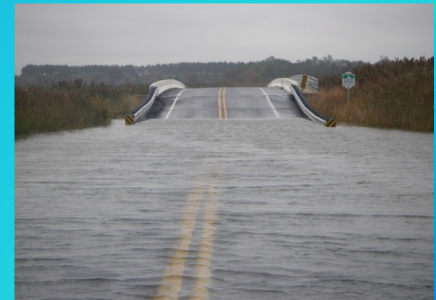
Daily Tidal Flooding – DE 9
