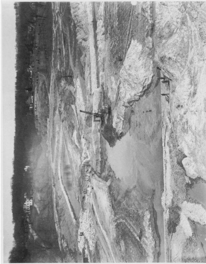
13. "WPA dredging and filling the Iowa River near the University of Iowa, April 1938." Work on the west bank was extensive. This picture was probably taken from the top of the university's Mabie Theater, looking north. The stone work in the upper left was part of the border of the future canoe pond that can be seen, finished, in photo #16. The pond was drained in the 1970s for the construction of the Music School, Clapp Recital Hall, and Hancher Auditorium. (State Historical Society of Iowa)
