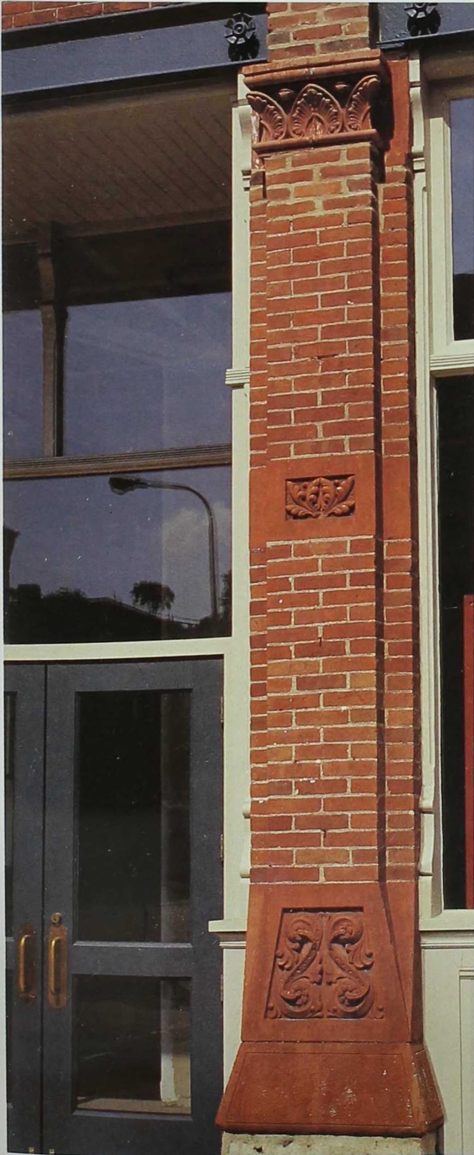
B rick piers, which define the bays on the west facade, are still ornamented with rich terra cotta detailing.
