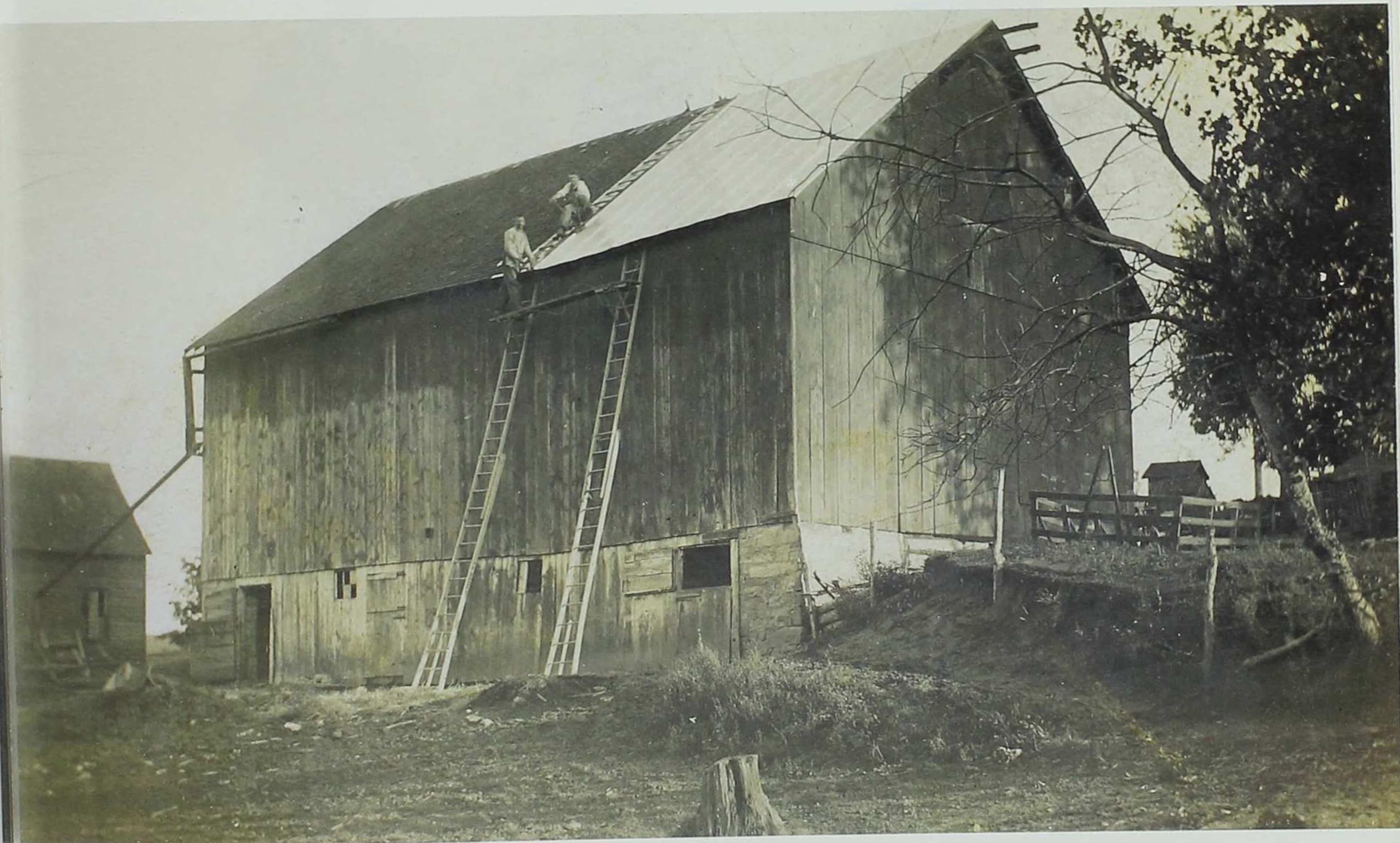
Left: Billy (hatless) and another worker take a break, surrounded by lumber and scaffolding at the building site of a new barn.
