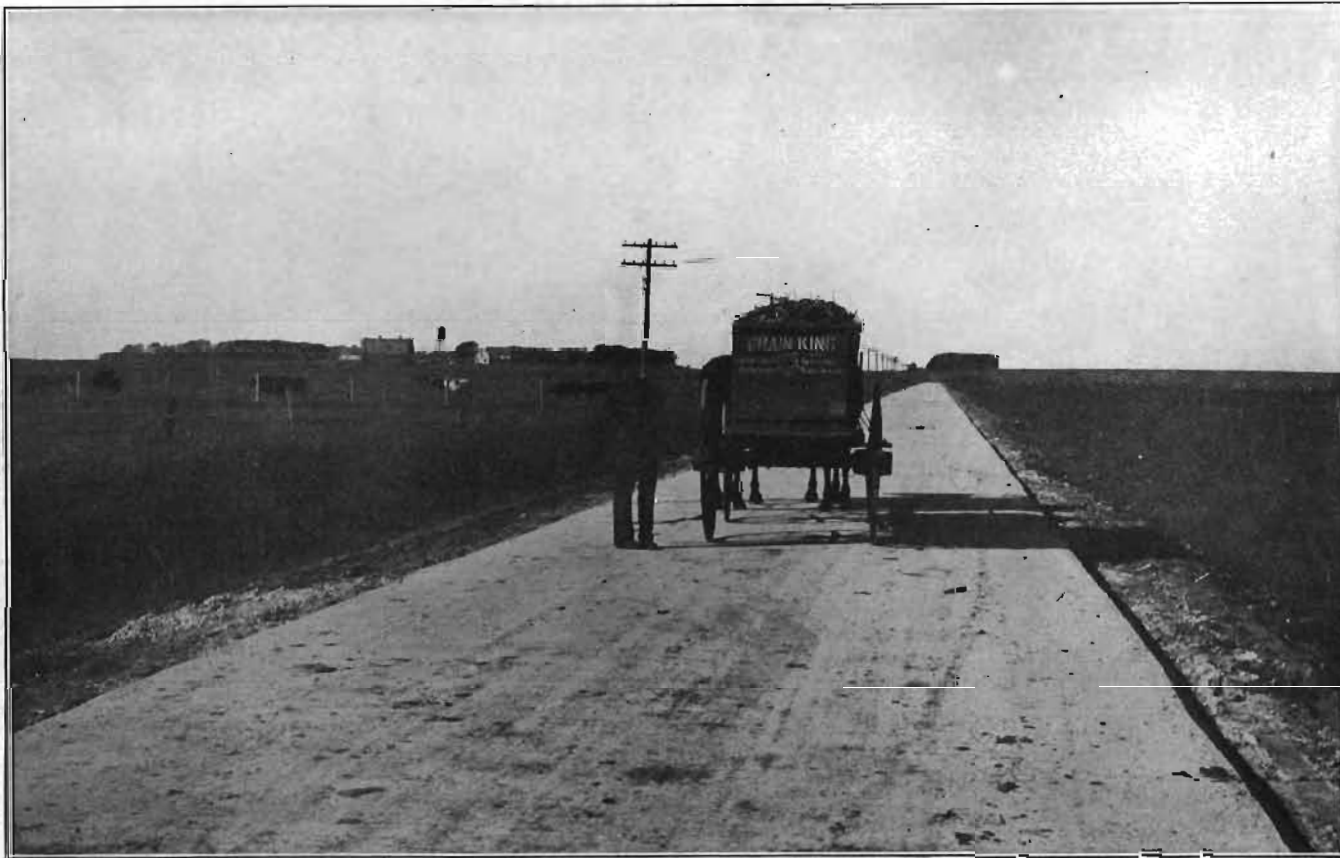
PLATE VII—Mason City-Clear Lake road after laying the concrete but before bank is done. Cerro Gordo county.
