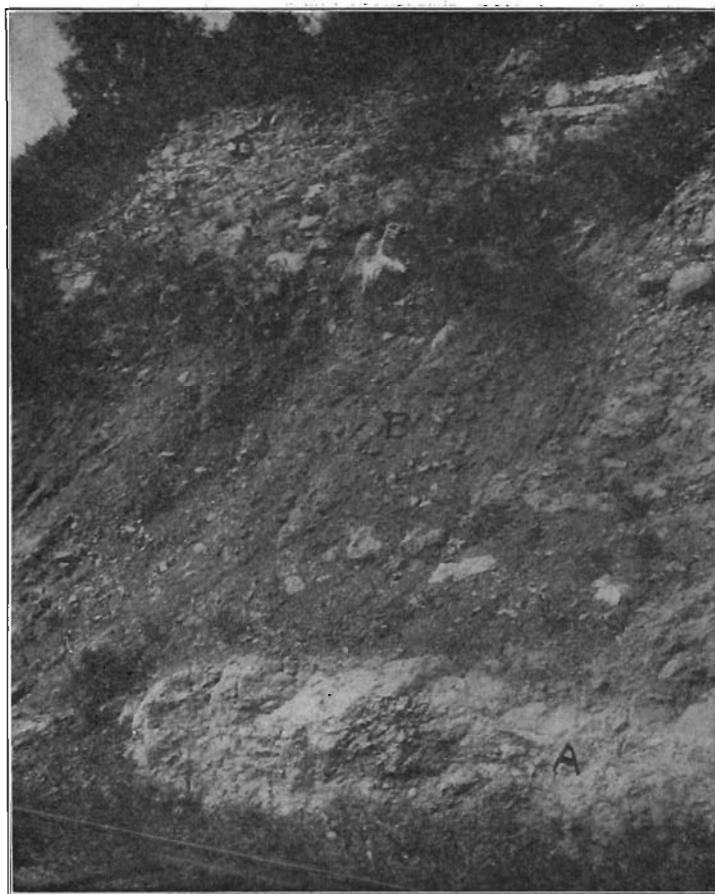
FIG. 65.—General relations of the Independence zone of brecciation. Railway cut north of Vinton, Benton county. A, Ledge of Otis calcilutite, brecciated. B, Independence zone. C, Upper Davenport beds, brecciated. D, Barren beds, arched, in places brecciated.
