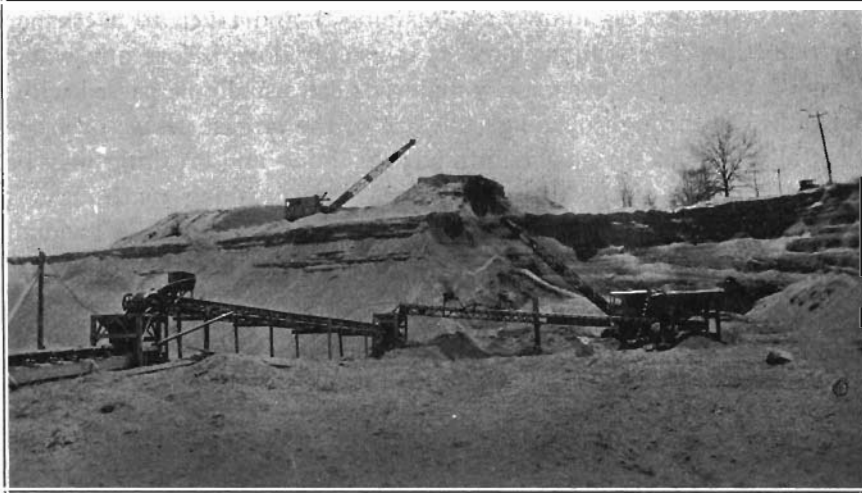
FIG. 29. — Bellevue Sand and Gravel Co., Bellevue. View of the Belt Conveyor System.
