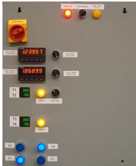
Figure 4. Heat exchanger control panel developed for manual/auto access.
