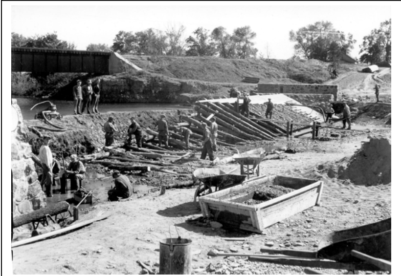
WPA workers construct a dam on the Shell Rock River near Plymouth in Cerro Gordo County during the Great Depression.
