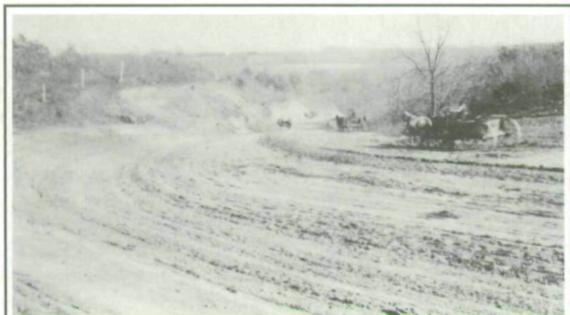
Workers grade Danger Hill with horse-drawn equipment in 1920. The "spectacular cut" is visible near the center of this view, as the curve sweeps down the hill. Remodeling the natural topography to fashion a gradual curve at Danger Hill represented a pioneering effort by the Iowa Highway Commission. The "cut," which lowered the road by as much as fifteen feet, was accompanied by a "spectacular fill" of twenty-seven feet at the bottom of the hill. Courtesy Iowa Department of Transportation.
